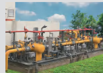
调峰站减压撬 Peaking Shaving Station & Pressure Regulating Skid
