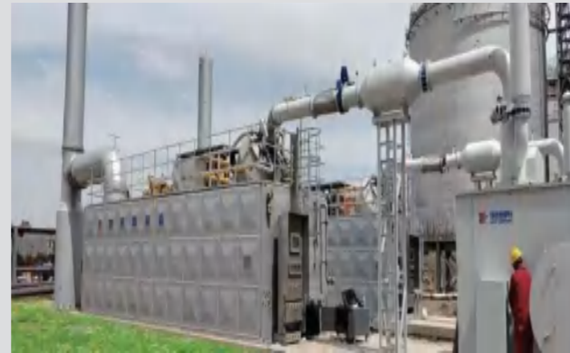
为西宁中油燃气提供2台浸没燃烧式气化器现场 Provide 2 units SCV on-site for China Oil and Gas in Xining
