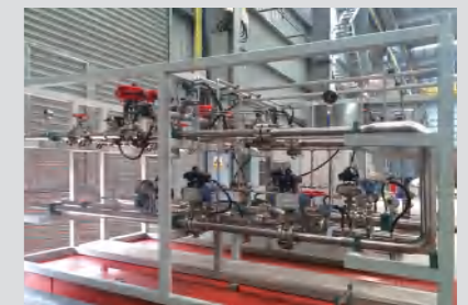
氧气、天然气混合撬 Gas Mixing Skid of O2 & NG
