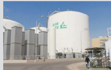
AP沙特吉赞项目空温式气化器现场 Ambient Air Vaporizer for AP Saudi Arabia Jazan Project
