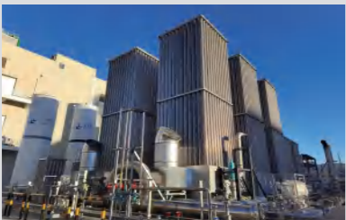
Linde空温式气化器现场 Jobsite of Linde Ambient Vaporizer
