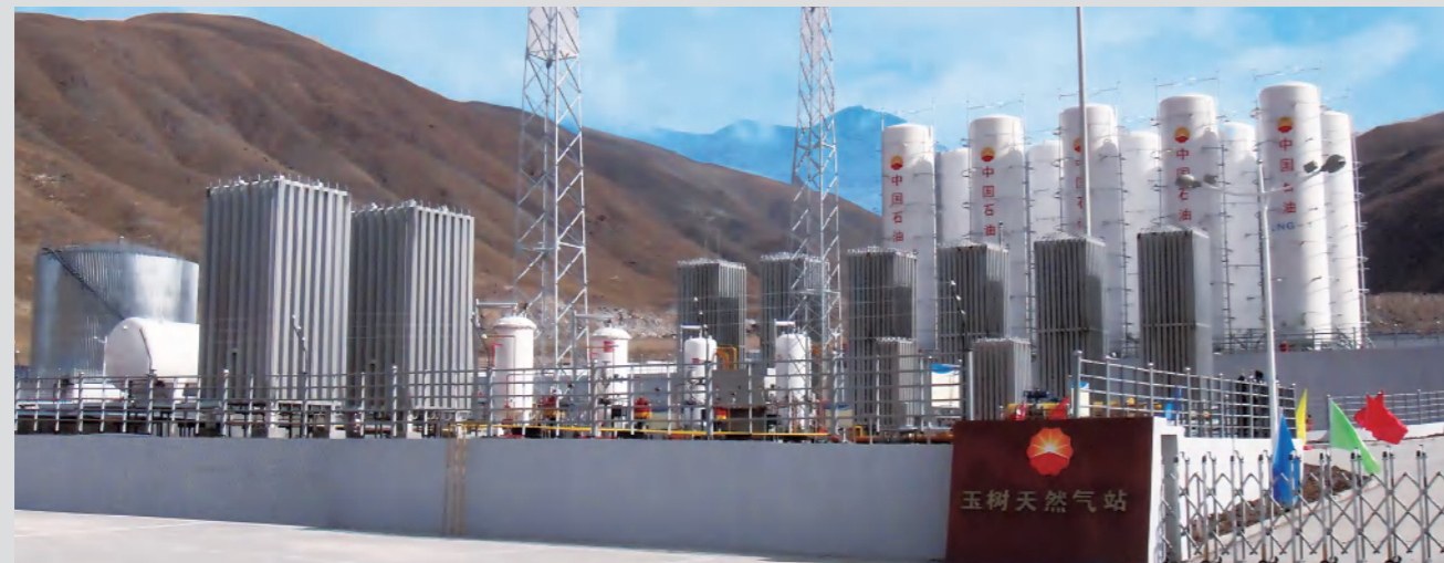
特莱姆为青海玉树灾区政府援建项目提供的 LNG、LCNG 气化器、加热器现场 LNG、L-CNG vaporizers and heaters' operating site of Qinghai Yushu disaster area government reconstruction project which provided by Wuxi Triumph
